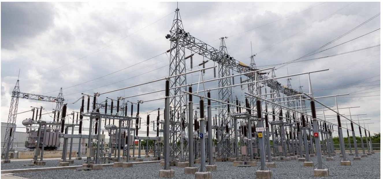
Image 5: Example of a 400kV Substation
